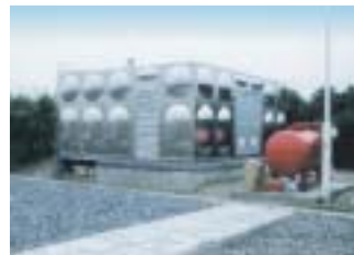
Fire-fighting water tank (Kyushu Factory)
