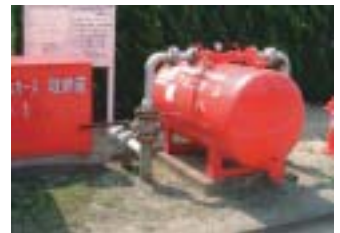
Fire-fighting water tank (Ohtake Research Center)
