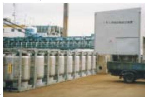
By switching to IBC, premise of the shipyards were much better put in order
