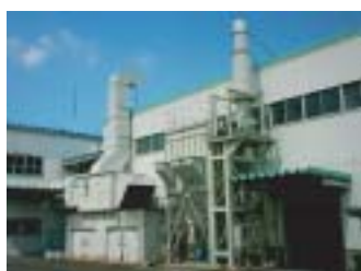
Dust collector (before) and air intake & exhaust equipment (behind)
